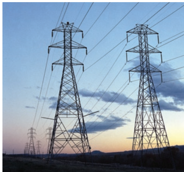
High voltage transmission lines
