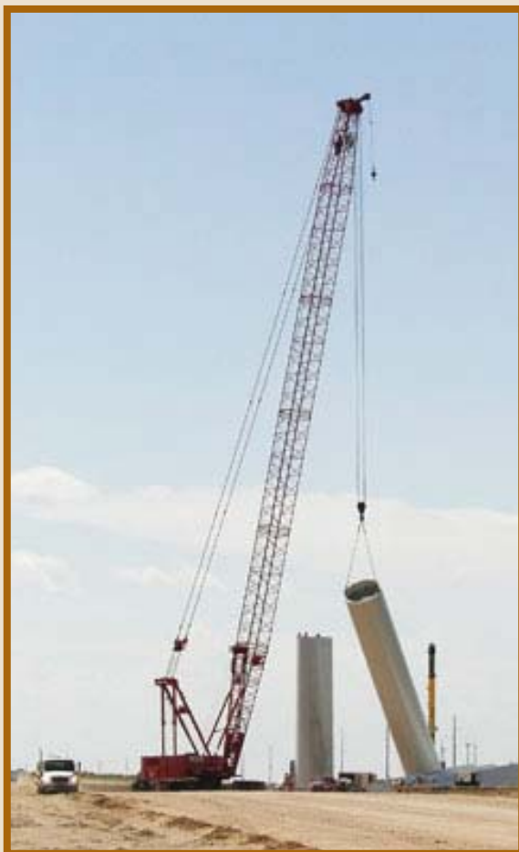
"These are the largest construction projects in the history of the county," said Rich O'Connell, director of the Logan County Economic Development Corp.
