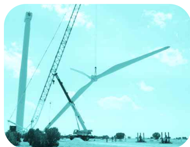
Public Service Company of New Mexico will be purchasing the output of this 204 MW wind project currently under construction near House, NM.
